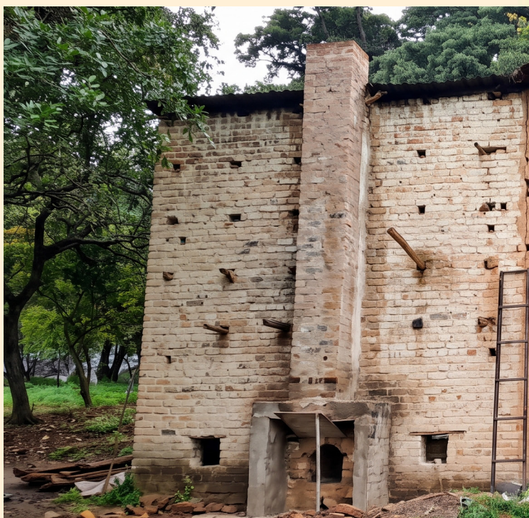
A chimney that extends at least 30 cm above the height of the barn roof.
